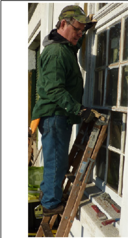
GETTING INTO A SCRAPE – Richard McNew scrapes before applying TLC to the baggage room window sash.
