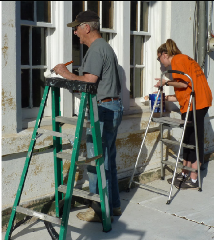
DRESSING UP THE DEPOT – Gary Watson and Debby O'Keefe handle the details of repainting the records room window sashes and sills.
