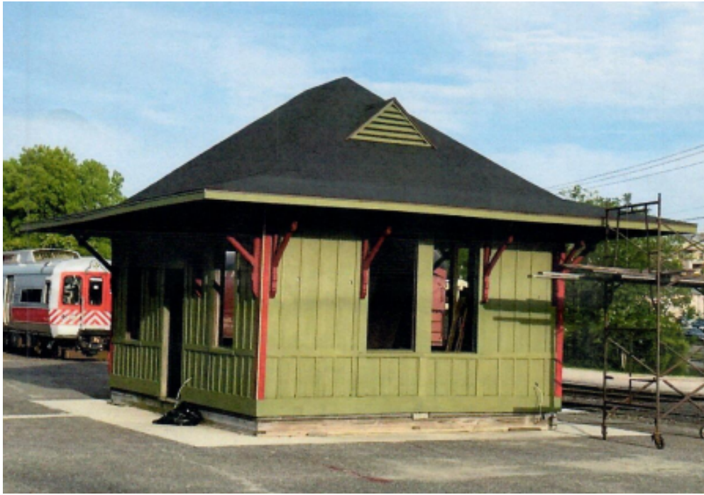
STATION ROOF AND BRACKETS INSTALLED AND ROOF COMPLETED - Grant money offset the cost of station canopy brackets, rafters and hip rafters.
