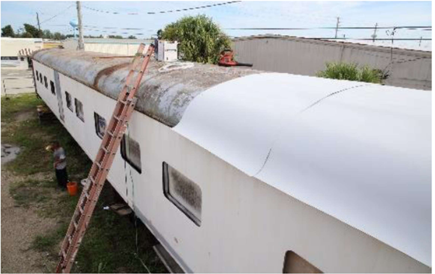
ROOF AND BODY WORK – Exterior repairs included replacing car sides and roof.
