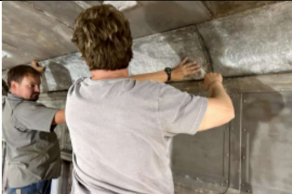
Volunteers Jakob Stage (left) and Michelle Yerkeson (right) fix and reinstall bent, corroded or missing panels.
