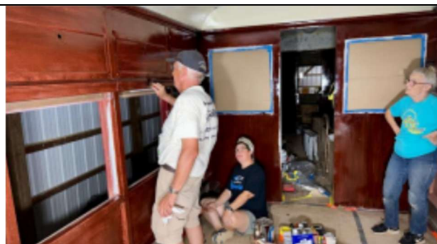
Volunteers Richard Witmer, Michelle Yerkeson and Lavonne Stage (left to right) apply and texture the first coat of stain.
