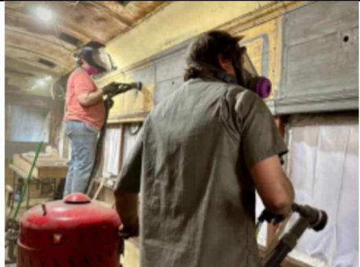
Volunteers Michelle Yerkeson (left) and Jakob Stage (right) wear respirators while slowly sandblasting all interior panels.
