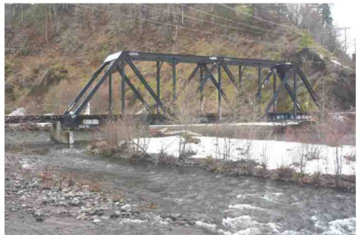
The relocated 1906 Warren Truss Bridge at Powerdale, which replaced a wooden Howe truss bridge in 1964. (Photo by T. Trent Stetz)
